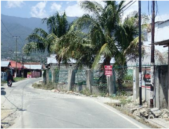
Fault movement affected community road to bend, Donggala Kodi
