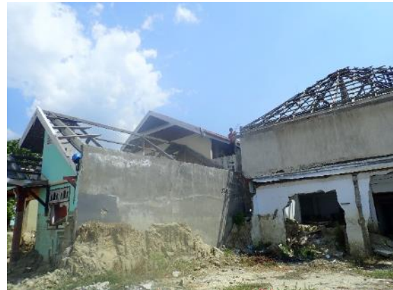
Mud flows developed by liquefaction damaged houses, Petobo
