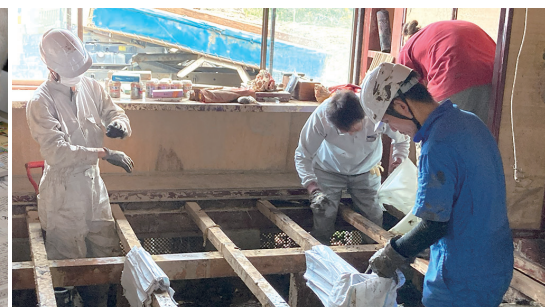
Volunteer activity for a flood-damaged house in Noto
